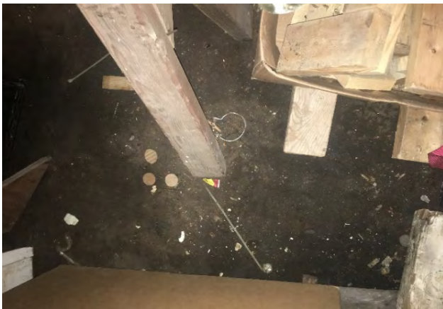
PHOTOGRAPH 15: Oil stained concrete floor below used oil tank drain.
