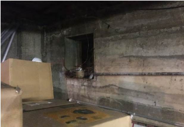
PHOTOGRAPH 7: Municipal water service entering basement.
