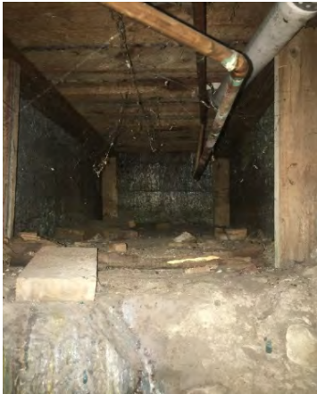
PHOTOGRAPH 13: Evidence of automotive paint running down wall in northwest corner of basement.
