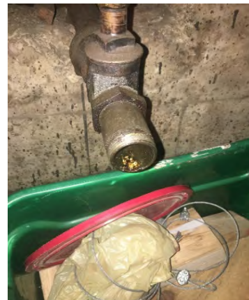
PHOTOGRAPH 10: Drain from used oil storage tank located in basement.
