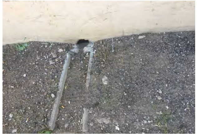
PHOTOGRAPH 2: Drain into alleyway from floor trap.
