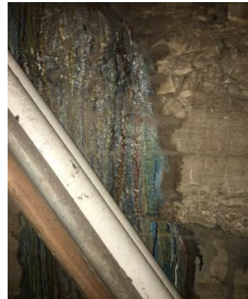
PHOTOGRAPH 14: Evidence of automotive paint running down wall in northwest corner of basement.
