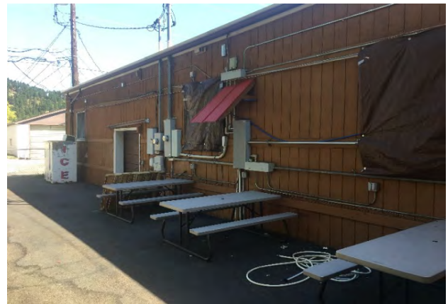
PHOTOGRAPH 4: Electric utilities near northwest corner of building.
