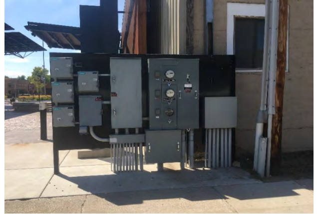
PHOTOGRAPH 26: Electrical panel near northeast corner for neighboring property.
