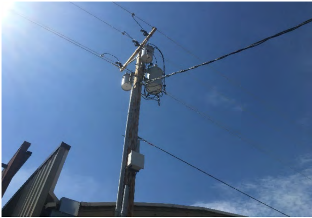
PHOTOGRAPH 27: Pole mounted transformer near northeast corner of property.
