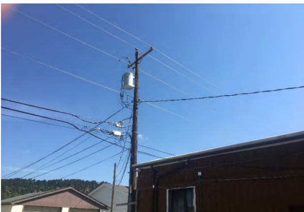
PHOTOGRAPH 5: Pole mounted transformer at northwest corner of property.
